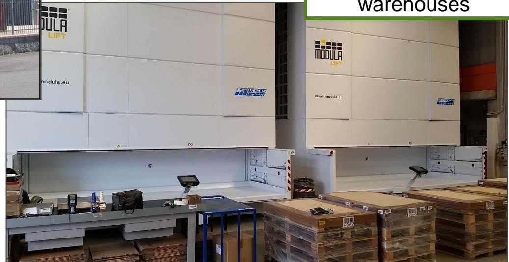
Automatic vertical warehouses
